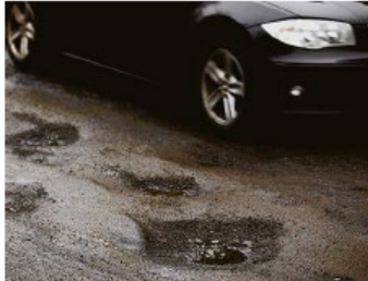
More than 100,000 potholes are estimated to have been reported in 2021
